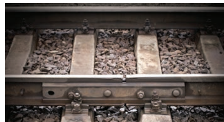
Figure 7.1 Gap in railway track
